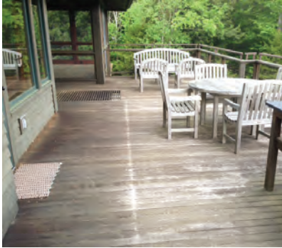
Located in the heart of Vermont's Green Mountains, this slope-side ipe deck hadn't been maintained since its installation 14 years ago. Note the drip line underneath the eaves.
